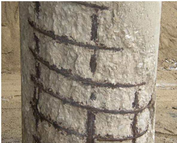
An example of corrosion caused by calcium chloride in concrete.
